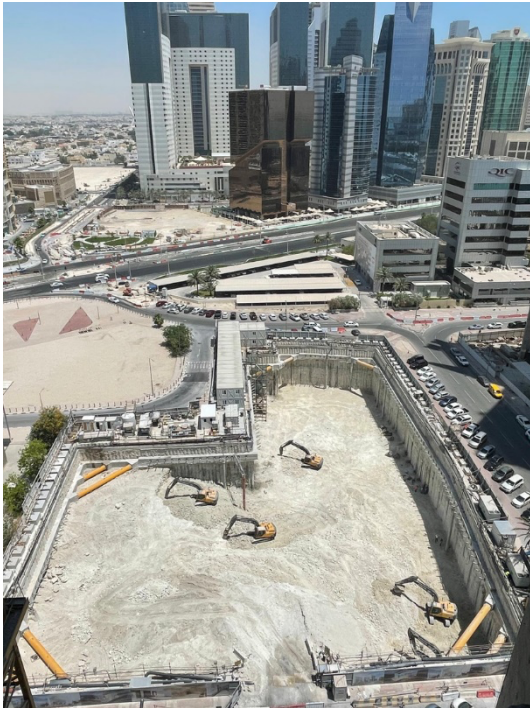
Fig. 12. Overview of the QP Multi-storey car park foundation construction showing lateral support system.
